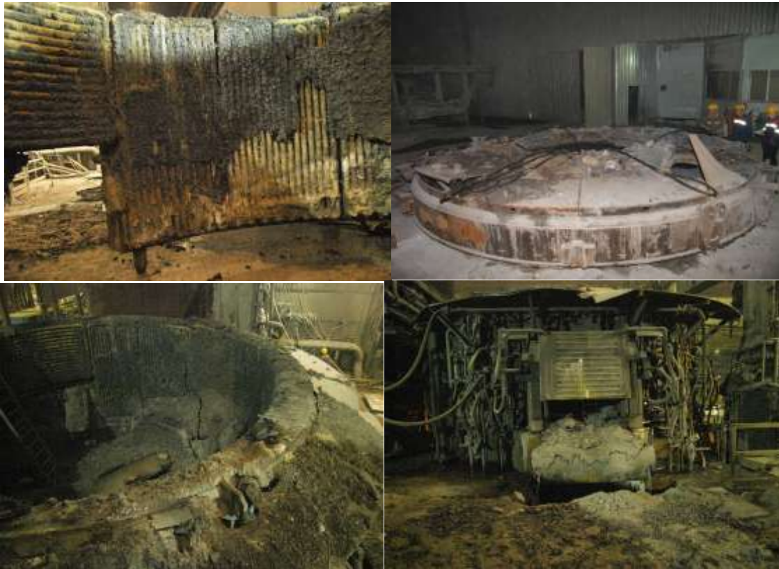
Figures 1÷4. Major damages identified in the EDP
