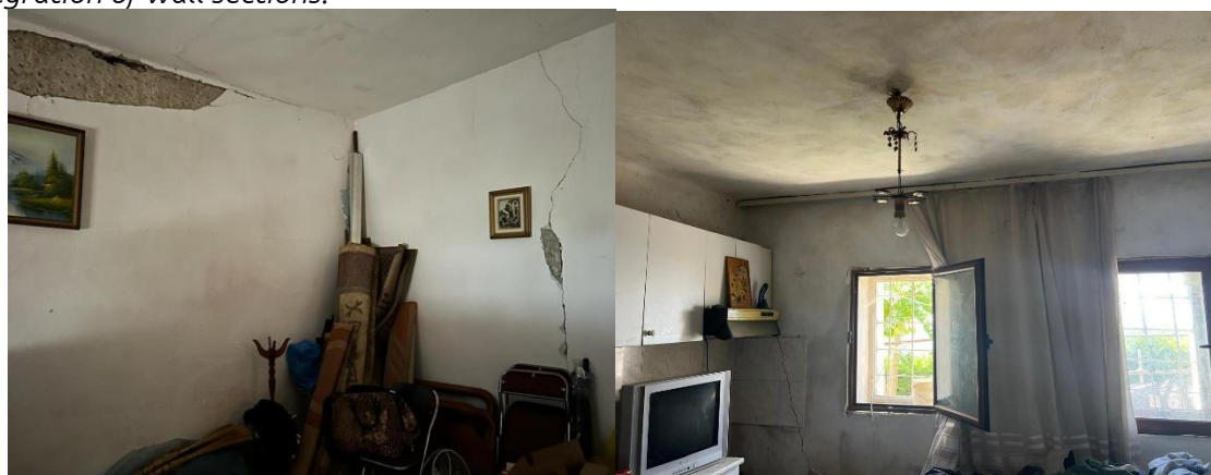
Figure 3. Damage patterns on stone masonry buildings
