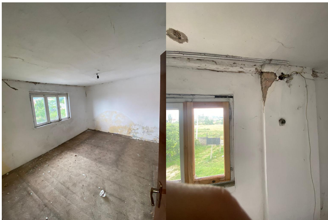
Figure 2. Damage patterns on brick masonry buildings
